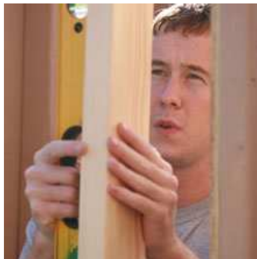
After gutting flooded homes in Cedar Rapids, Kerr helps reframe damaged walls.
